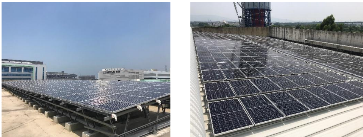
Photos of Rooftop Solar Power Systems
